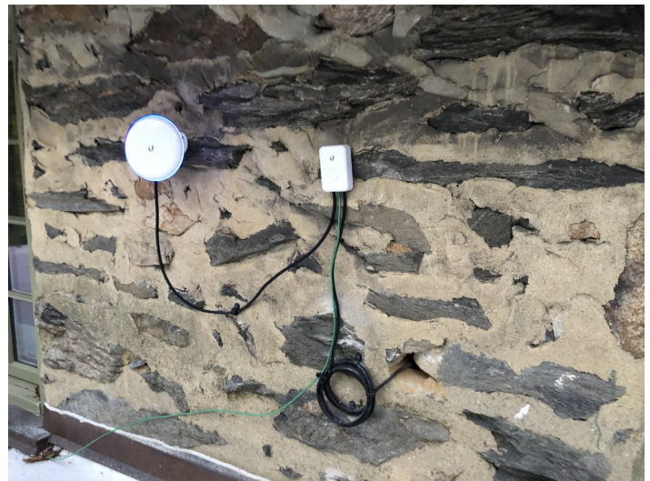
Transceiver dish and ethernet lightning arrester on the house
