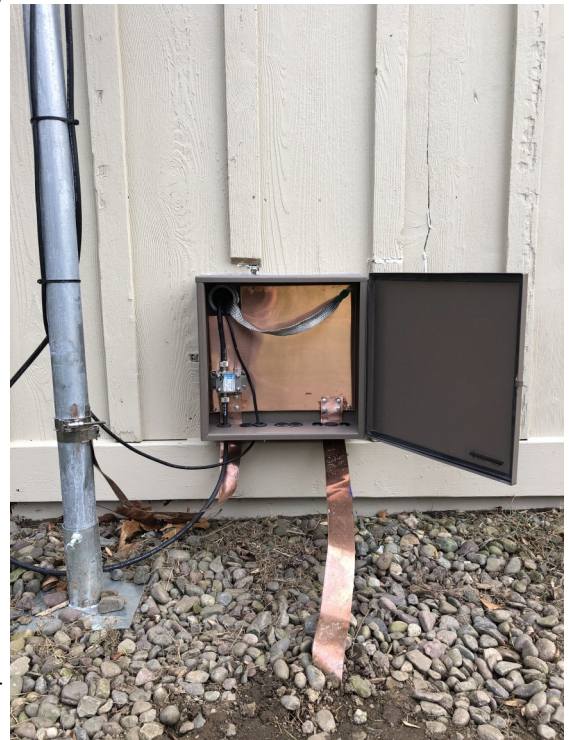
Entrance panel box in place with coax on lightning arrestor, ethernet from UBB (see below) to switch and tinned copper braid from station ground bar. I installed this medium size box to support future expansion to an HF RMS gateway and a remote wideband SDR and discone antenna. Perhaps I'll put other radios out here too.
