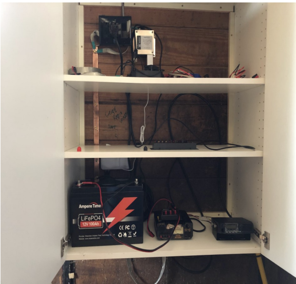
Ikea cabinet encloses power at top; vertical ground bus at left and provides space for the Winlink Gateway Station, backup power and future expansion
